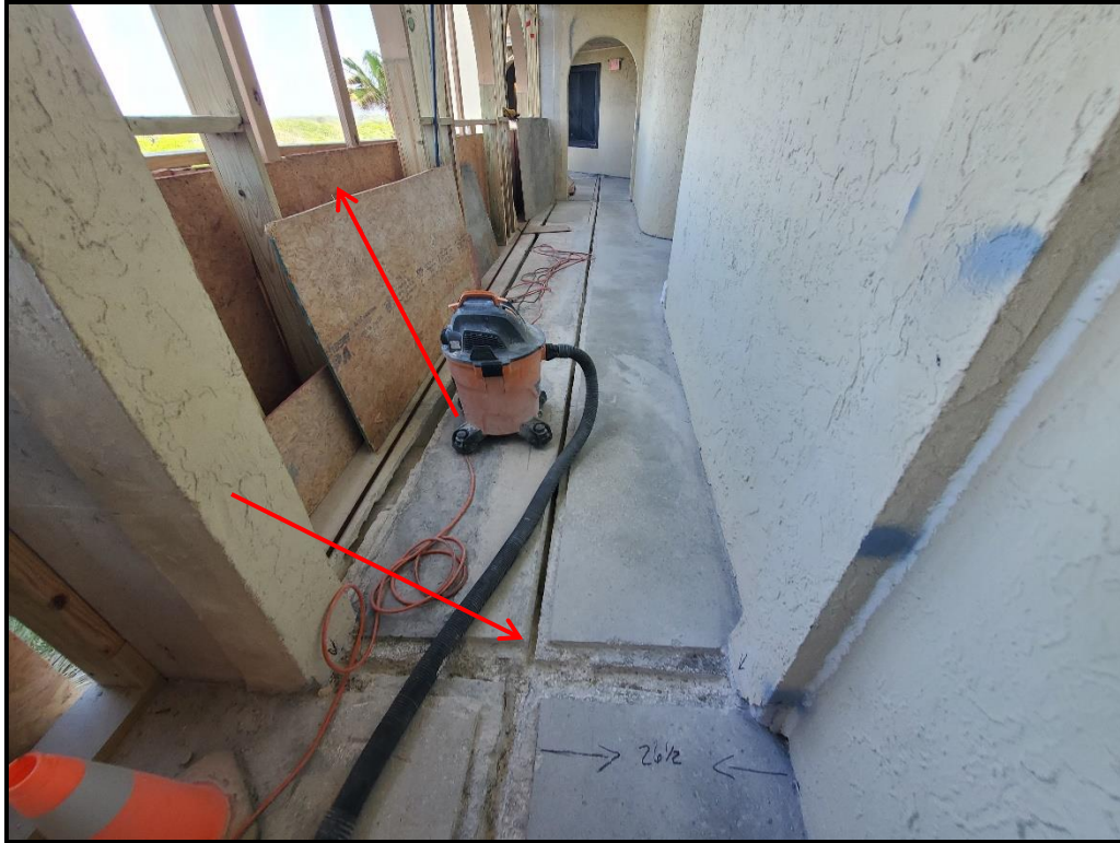
Photograph 2. 6 th floor archway sheathing installation and hollow core seam repairs in progress.
