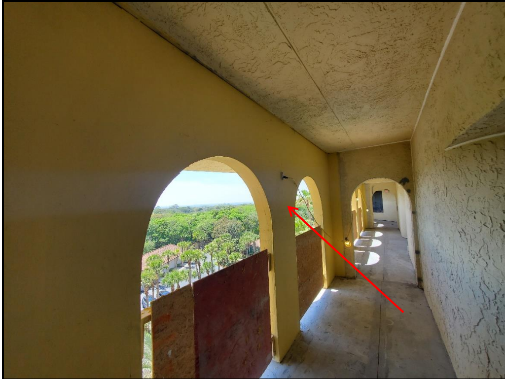
Photograph 10. 6 th floor archway rebuilds nearing completion, fluid applied weather barrier application in progress.
