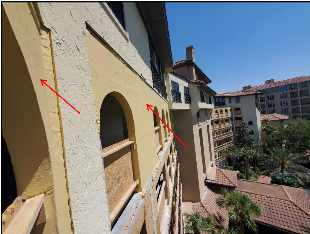
Photograph 9. 6 th floor archway rebuilds nearing completion, fluid applied weather barrier application in progress.
